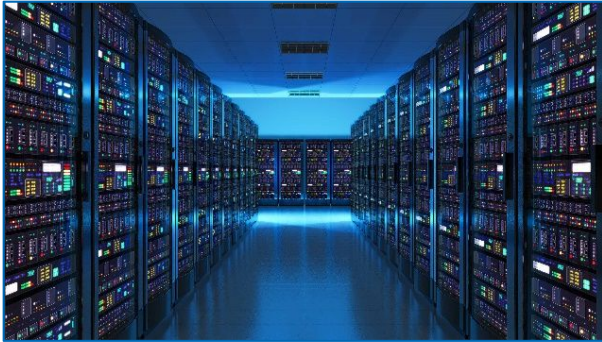
Uninterruptible Power Supply (UPS)
